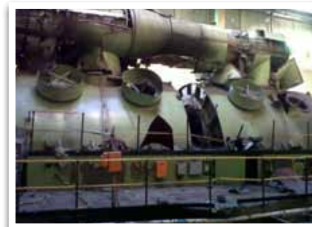
Figure 1: The Damaged Turbine
