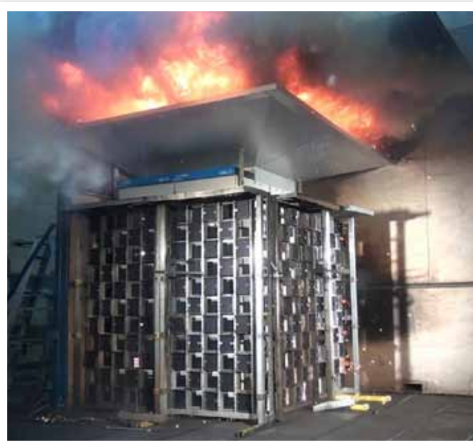
This picture shows the 31,5 kA/1 sec IAC type test on ACTOM MV Switchgear’s new AMV12 switchgear in progress at the KEMA test facility in Holland in September 2014.
