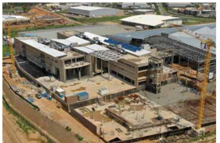
Longmeadow under construction. The additional 5 500 m 2 is being added to cater for expansion since the project began.
