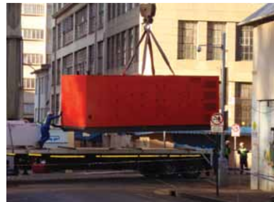
The Meissner generator is lifted off a flat-bed truck before being hauled over a five storey building and lowered into a basement where it will spend the rest of its days.
