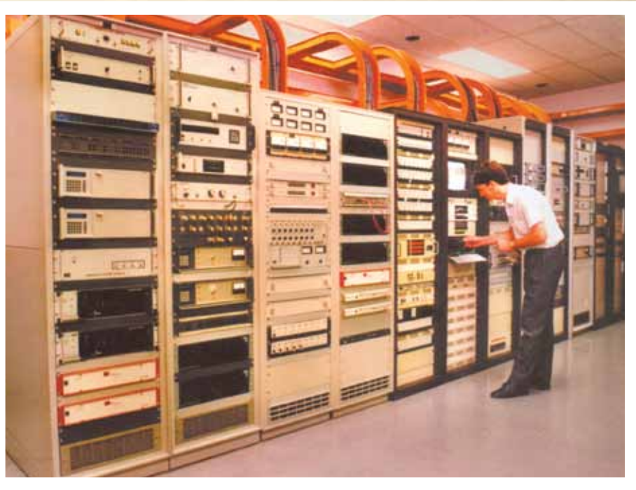
Satellite uplink and downlink equipment.
