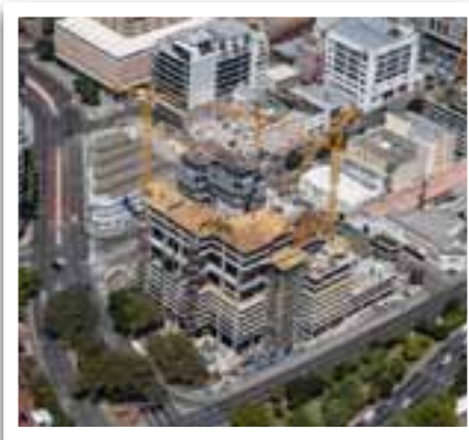
An aerial view of the Portside project which is being undertaken by Murray & Roberts, Western Cape.
