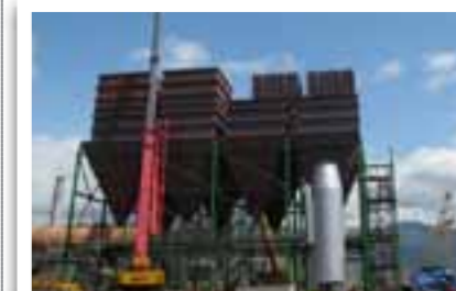
The rotary dryer bag house for the Lion Ferrochrome expansion project as seen in February 2013 while in the process of being erected, showing the bag house casings and dust collection hoppers mounted on the support structure.
