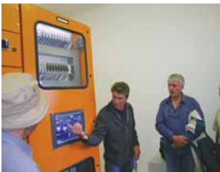
Management and control system being explained.
