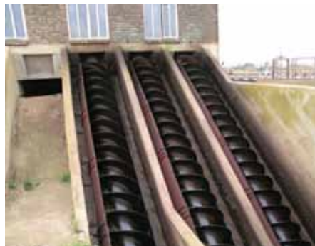
Spiral pumps lifting water to be aeration dams.
