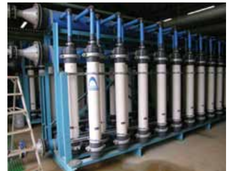
Ultra filter skid – three skids installed side by side.
