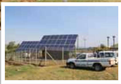
SAPS Katkop - Staggered Array
