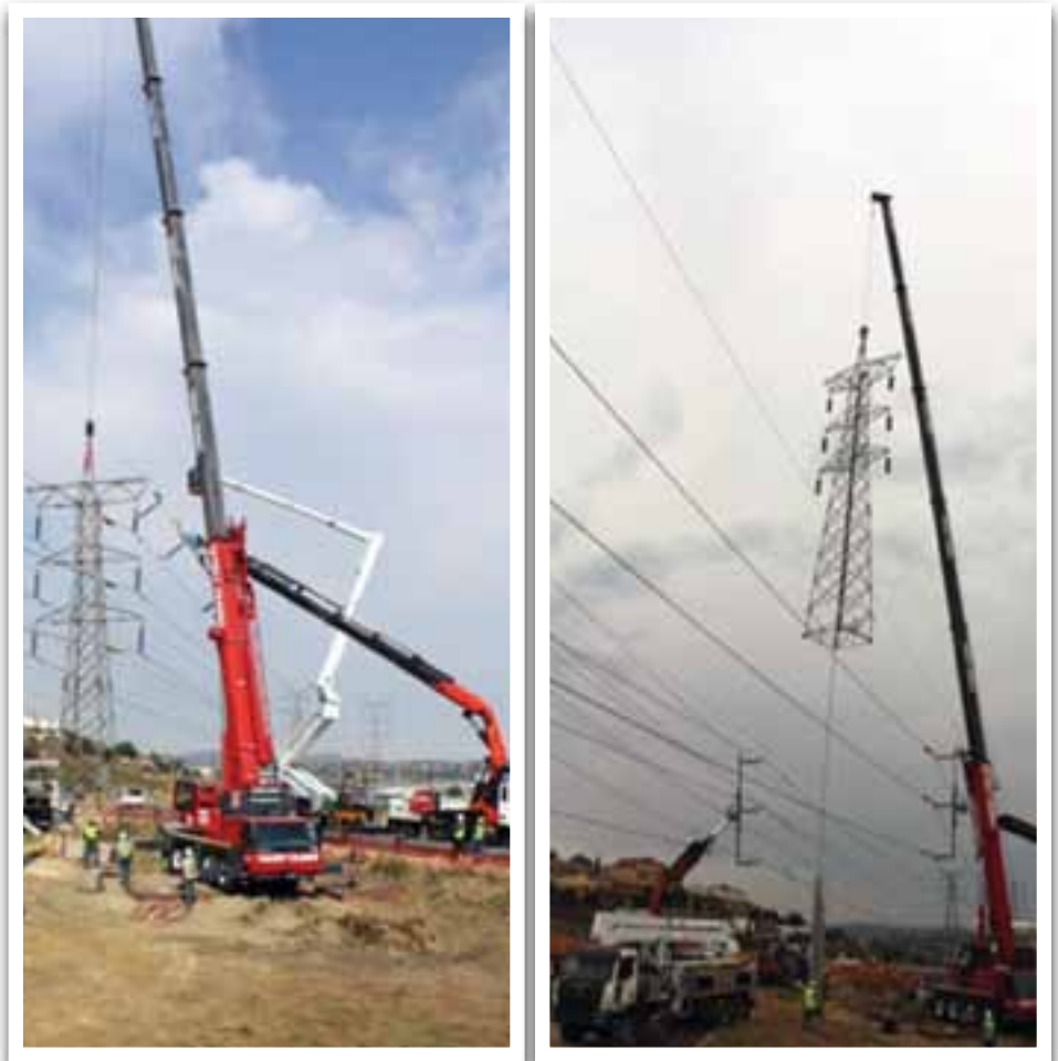
Damaged tower being removed while conductors are still energized
