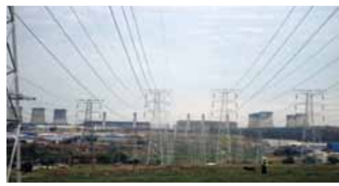
Kelvin to Cydna 88kV transmission lines
