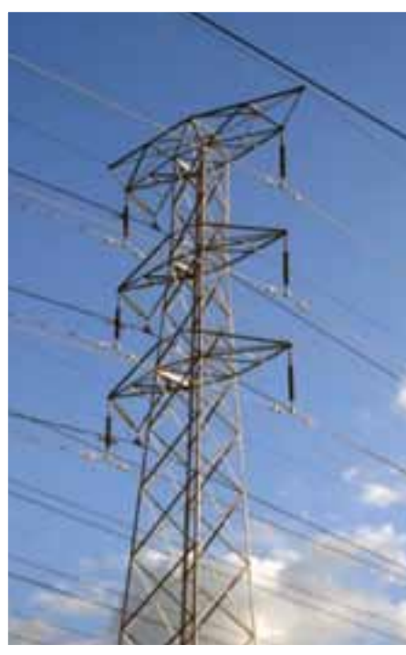
Bypass conductor in position to allow load transfer from conductor to be replaced
