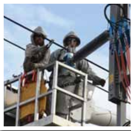
Live-line worker touching a wand to the live conductor to be at the same electrical potential as the line voltage
